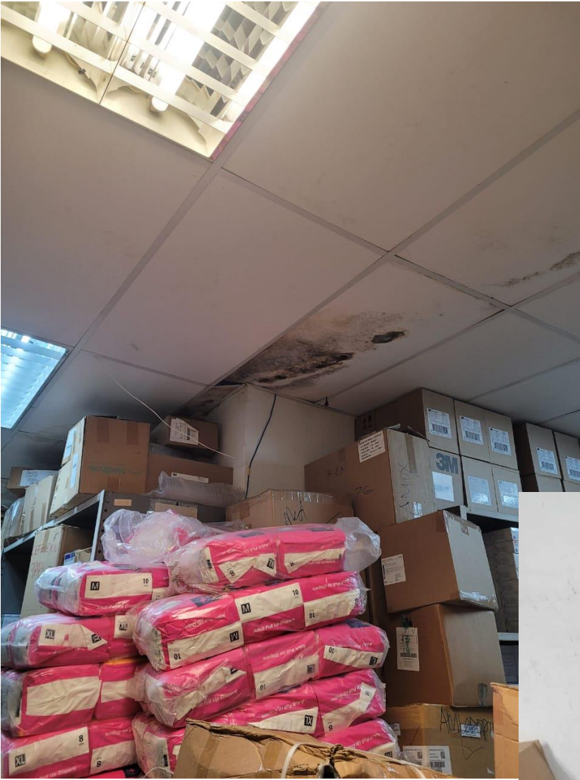
Picture 13: Water leaked on the pharmaceutical products.
