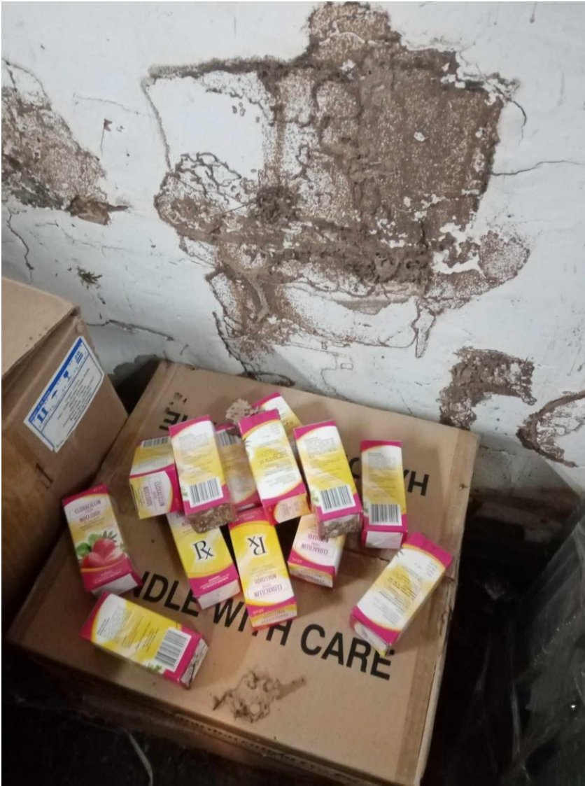
Picture 10: Inside the Pharmaceutical Storage, children medications were damaged from termites.
