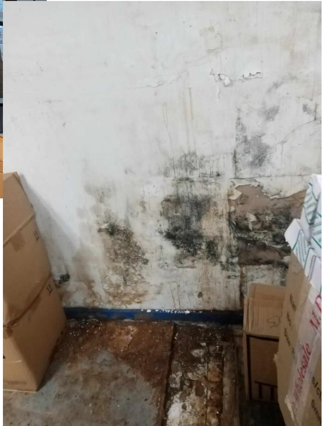
Picture 14: Mold was accumulated in the Pharmaceutical storage room.
